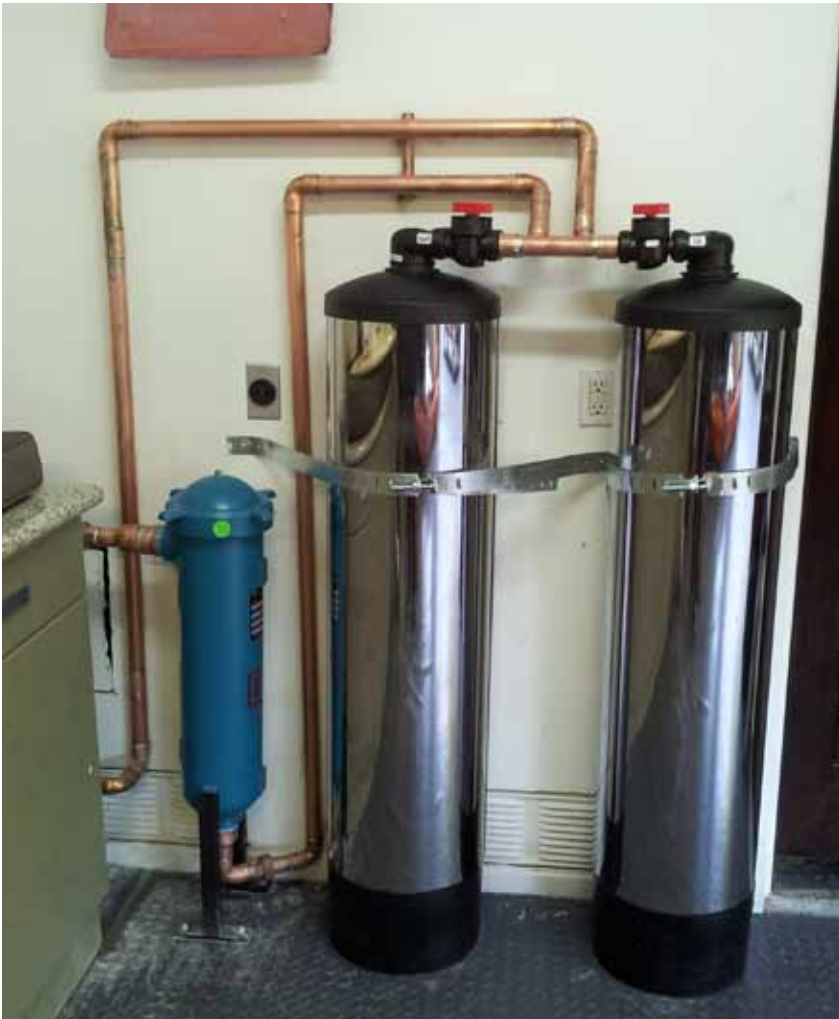
2-1/2 cu. ft. installation with large sediment filter (stage 1) inside garage
